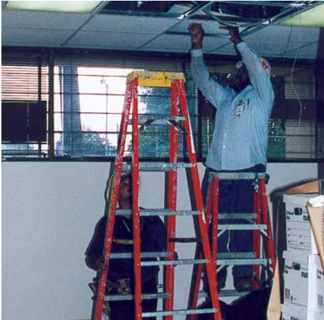
Flood repair at the Stehlin Foundation
